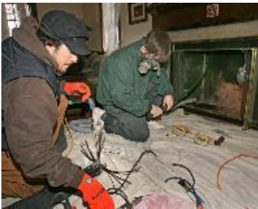
Karl Ramirez (left), owner of Ramirez Restoration, and employee Nathan Dunkelberger clean soot from a Wauwatosa chimney this week. Ramirez said of the Emerging 200 program: "It helped me to set some goals up through 2012 and helped me to see the potential for growth."
